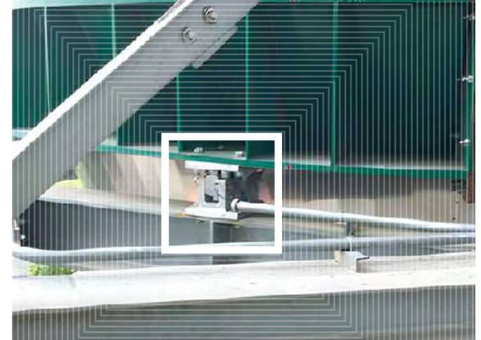
3. high capacity silos
